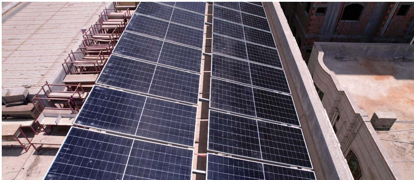
The solar system YFCA installed for the school.
